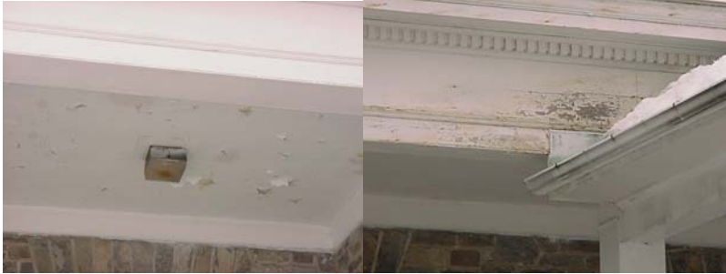
Remove loose paint and recoat.
